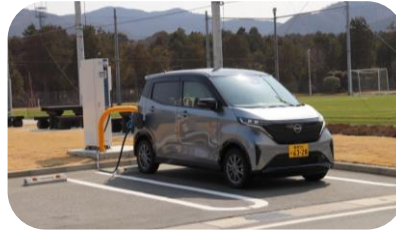
EV charging station
